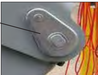
No rust. Pin has not rotated. Area is clean of dust/metal shavings
